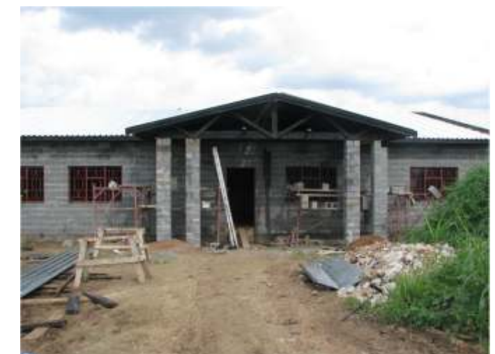
The new Buseko Home now has a roof and we have begun the finishing process
